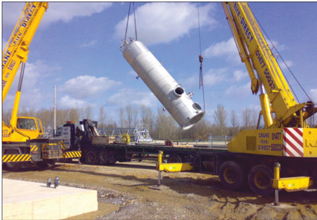
The first reactor, which was prefabricated off site, is lifted into place
