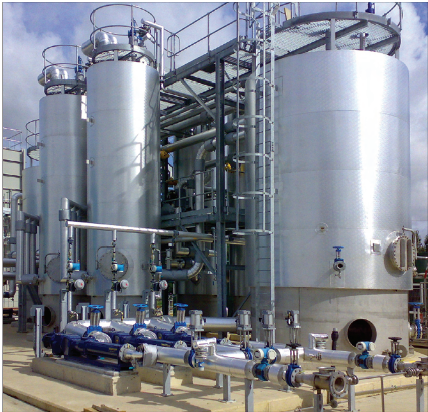
The new thermal hydrolysis plant at Cotton Valley Sludge Treatment Centre in Milton Keynes is ready for commissioning
